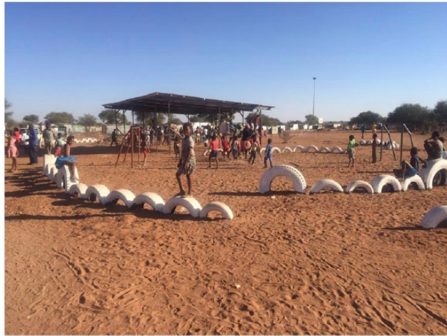
PHOTOS 3A AND 3B Construction (A) and finished (B) public space in Freedom Square
